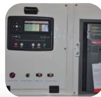
Control Panel & MCB
